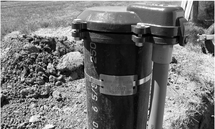
A well tag, displaying the well identification (ID) number, should be on every well.
